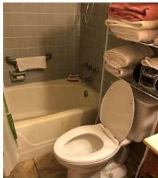
new higher UD toilet
